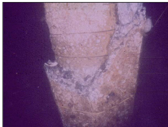
Figure 3-25 Pile Damaged by Delayed Ettringite Formation
