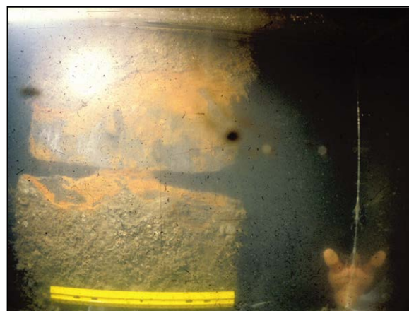
Figure 3-27 H-pile Corrosion Below Concrete Encasement
