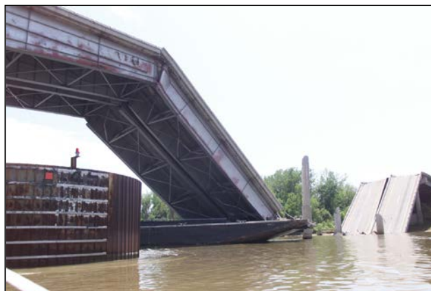
Figure 1-6 Vessel Impact Damage at I-40 Bridge over Arkansas River, Oklahoma (2002)
