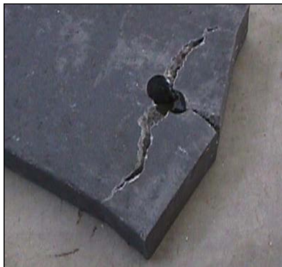
Figure 3-39 Failure of Composite Member
