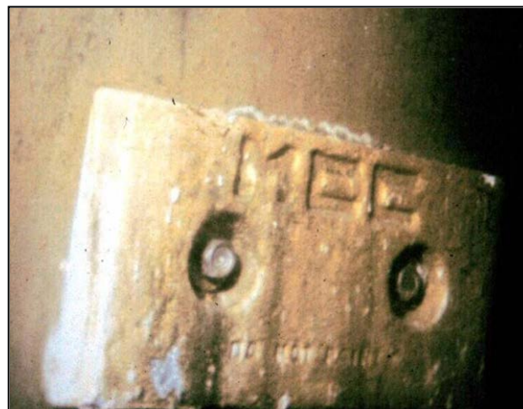
Figure 3-33 Sacrificial Anode on Steel Pipe Pile
