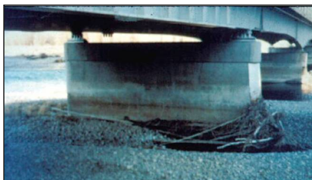
Figure 6-8 Upstream Scour Hole and Debris with Downstream Deposition of Material Shown in Dry
