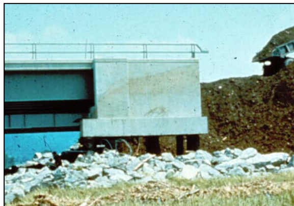
Figure 3-4 Exposed Timber Piles at Scoured Abutment
