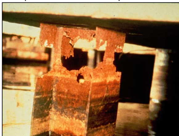
Figure 3-26 Severely Corroded H-Pile
