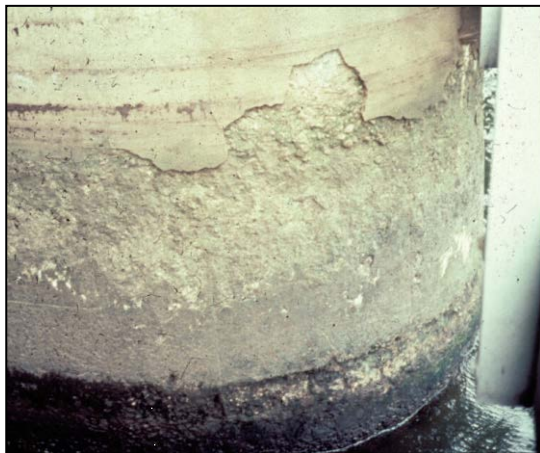
Figure 3-22 Scaling of Pier at Waterline
