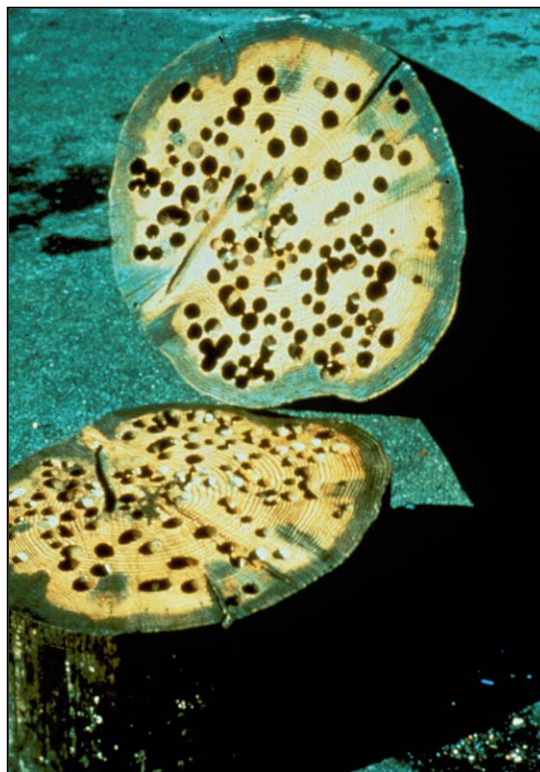
Figure 3-36 Timber Pile with Teredo Damage
