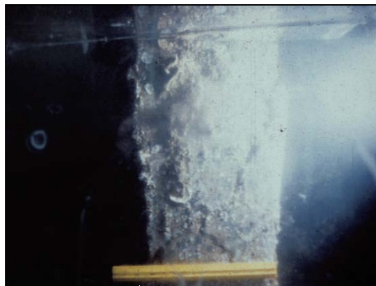
Figure 3-21 Cracked Concrete Pile
