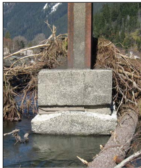
Figure 3-14 Foundation Seal Under Pier Exposed by Scour
