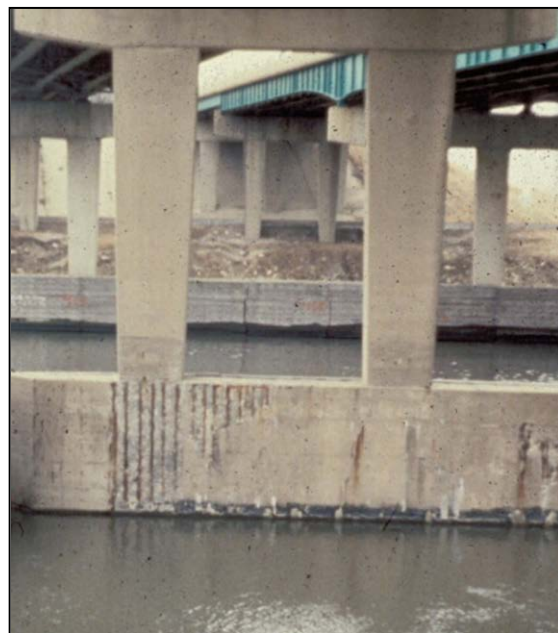
Figure 3-23 Spalling of Concrete at Waterline
