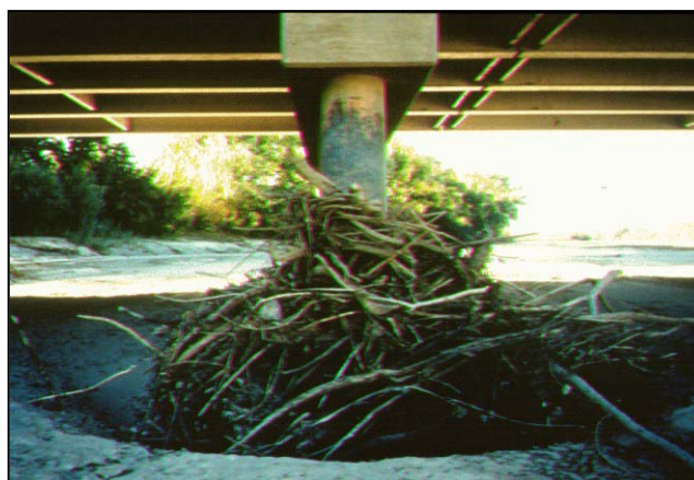
Figure 6-9 Debris Increasing Width of Pier
